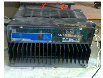
Fig.19 solar Inverter used.
