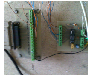
Fig.17 Data acquisition connected to computer
